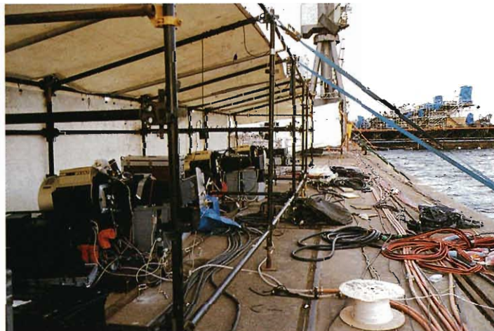
A dockside canopy for the fleet of Ludwig Pani BP6 Gold projectors.
